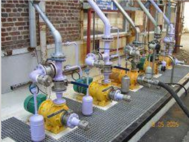
TANKER OFFLOADING PUMPS
